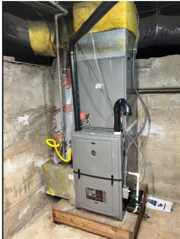
HVAC at Little House
